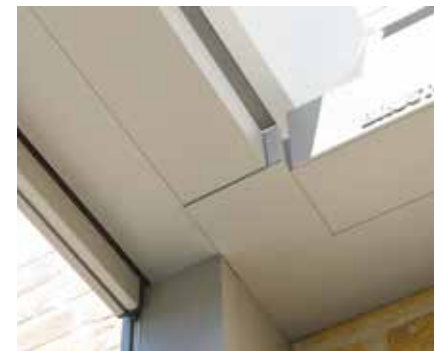
Water drainage through the gutters directly into the supporting posts
